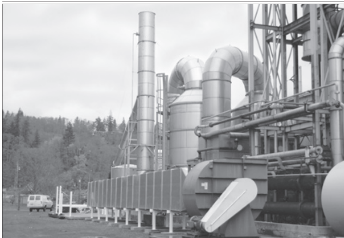
Ocean Protein’s towers scrub odorous compounds
